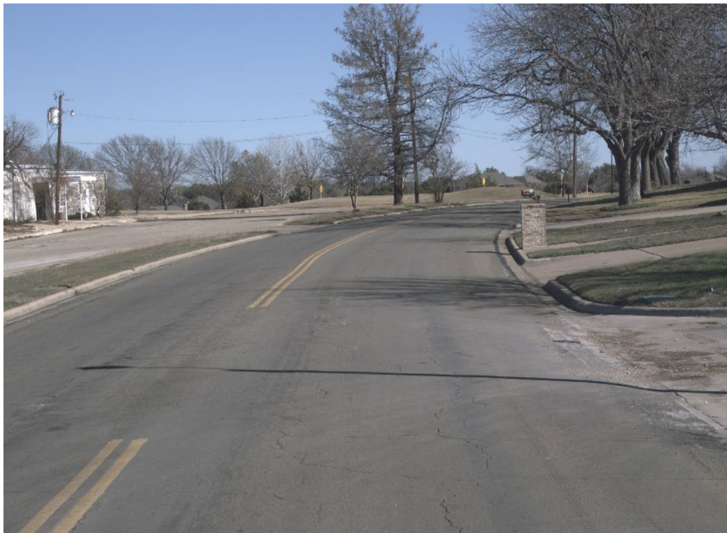
Figure 16: S ROY REYNOLDS DR (PCI= 38.1, Very Poor Condition)
