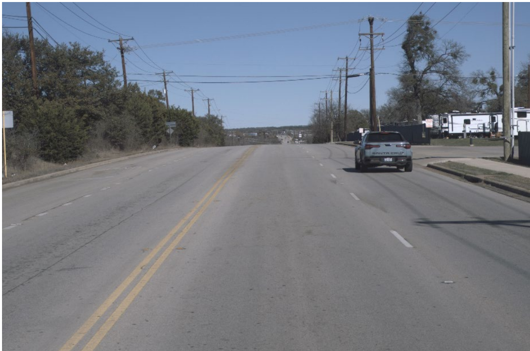
Figure 8: N ROY REYNOLDS DR NB (PCI=89.1, Good Condition)
