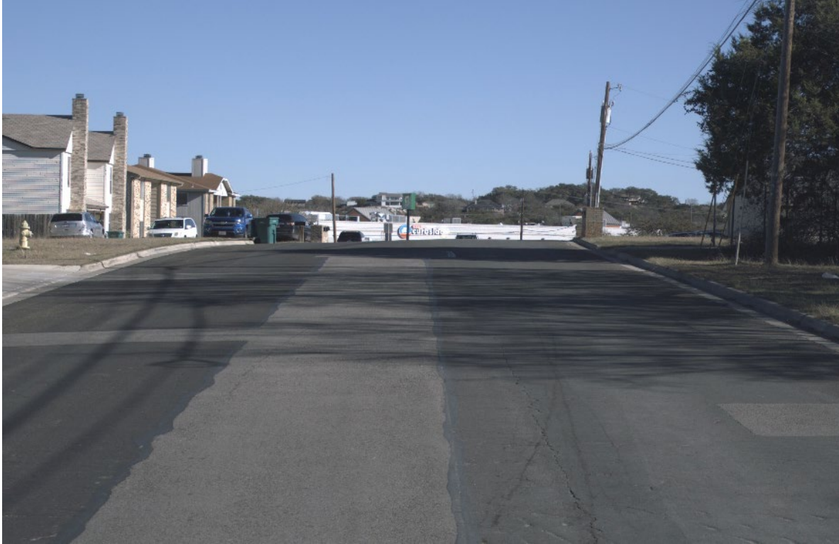
Figure 11: E BEE LINE LN (PCI=69.2, Fair Condition)
