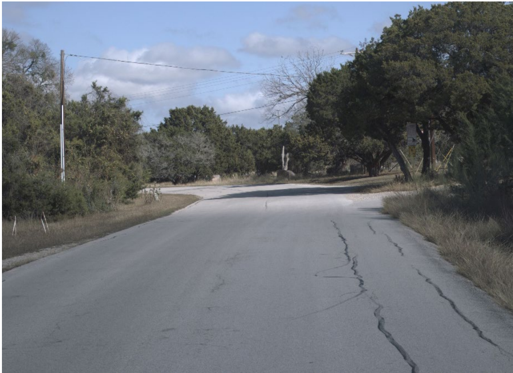
Figure 12: OAKRIDGE BLVD (PCI=60.5, Fair Condition)
