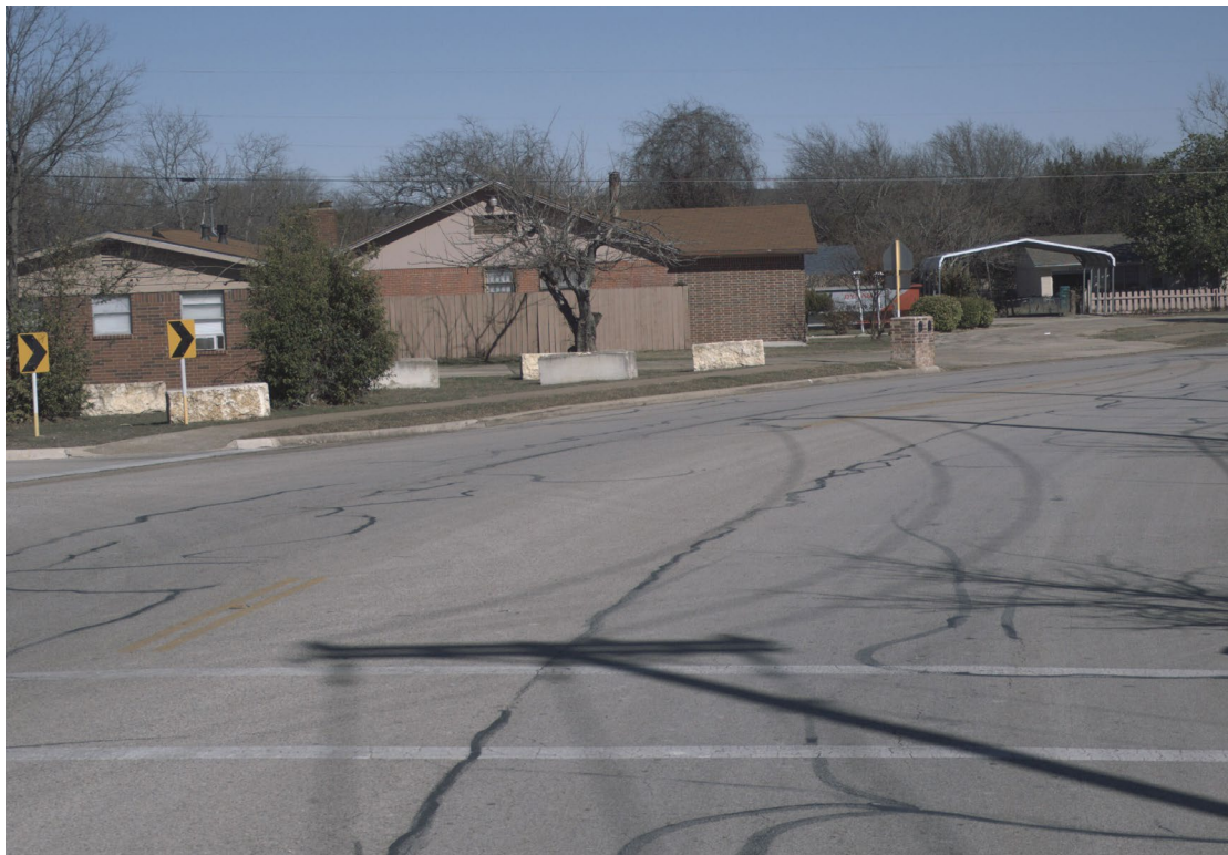
Figure 14: S ANN BLVD (PCI= 43, Poor Condition)
