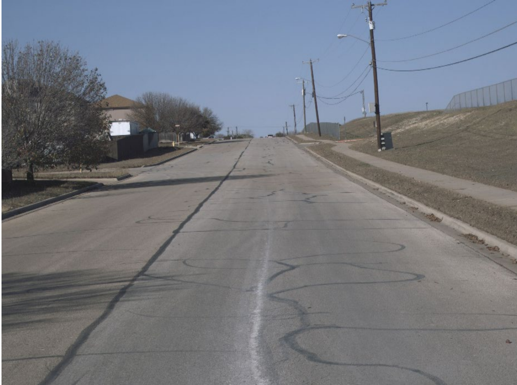
Figure 13: MODOC DR (PCI=46.2, Poor Condition)
