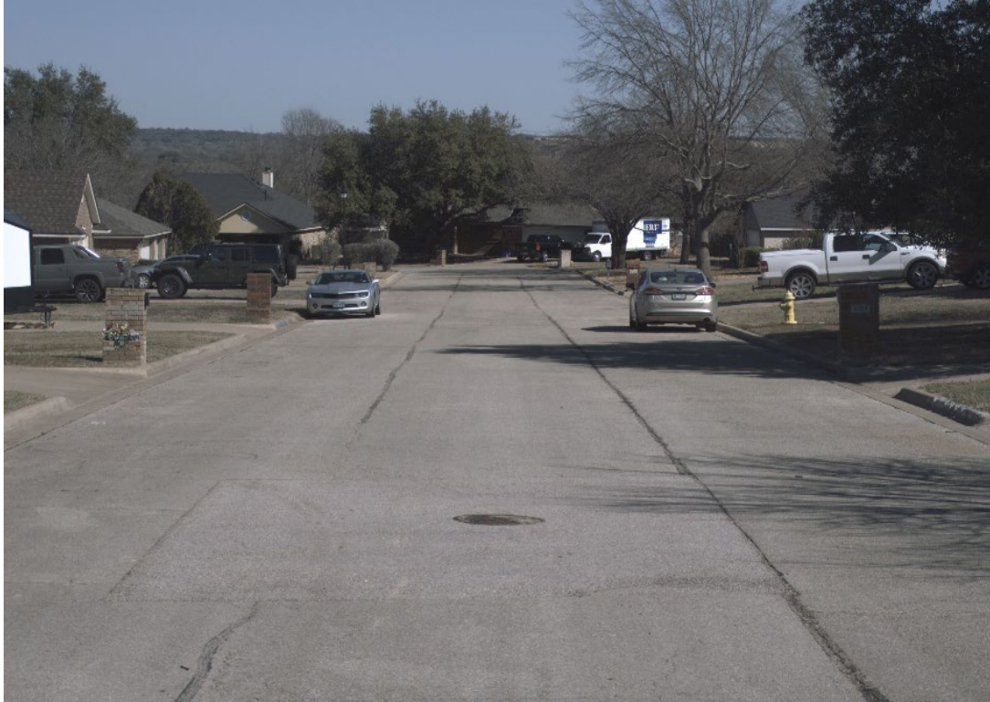
Figure 15: CITATION LOOP (PCI=29.2, Very Poor Condition)
