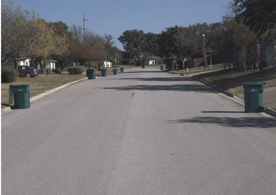
Figure 9: CATTAIL CIR (PCI=79.4, Satisfactory Condition)
