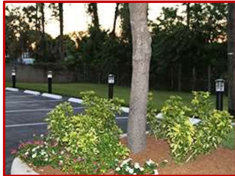
Figure 53 - Bollard Parking Lights
