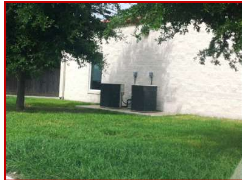
Figure 83 - Unscreened Service Areas are Prohibited
